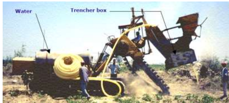
Figure 2. Spraying the trencher box with water to reduce friction with the soil
